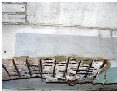
再劣化事例 Example of Macro-cell Corrosion
